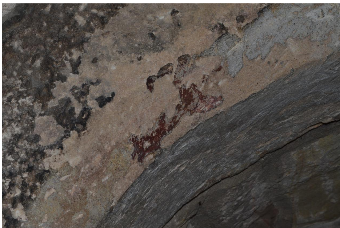
Trace of red paint in the chancel, on the chamfer of the western side of the arch over the north door.
