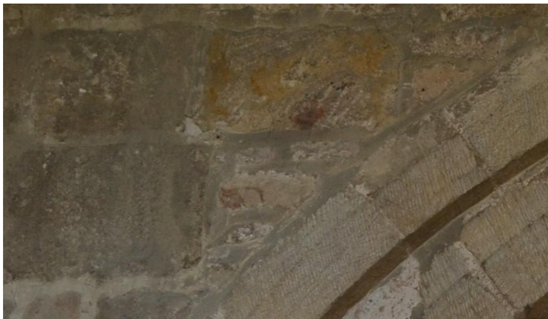
Traces of paint over the south side of the chancel arch, looking west from the chancel.
