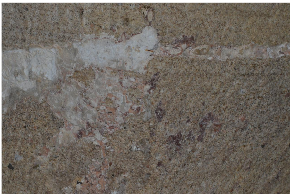
Closer view of traces of pink and red paint on the SE and E faces of the western pier of the south arcade. Photo looking north west.
