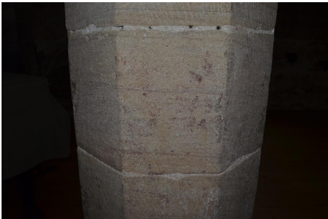
Traces of red paint on the eastern side of the eastern pier of the south arcade. Photo looking west.
