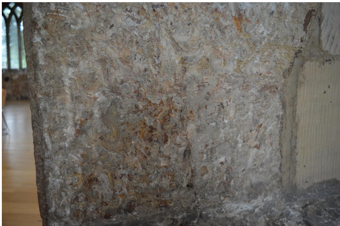
Traces of yellow and red paint on the hacked off masonry of the western side of the squint in the south side of the eastern respond of the south arcade.
