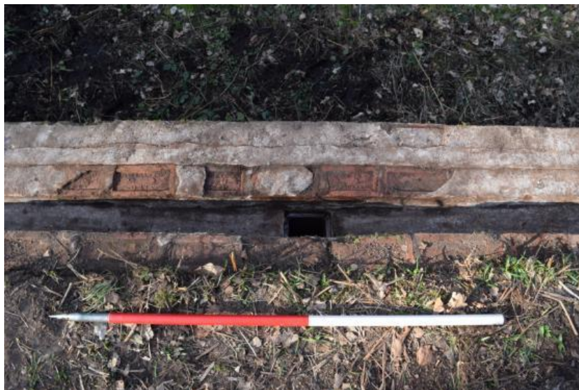
Photograph N_3: Overflow system. Southern wall of Immersion tank. An integrated mortar channel sloping from left and right into a grate in the centre.
