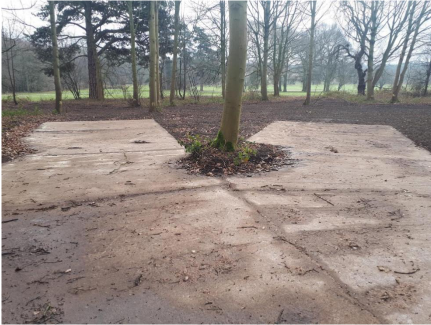
Photograph I_1: Concrete hard-standing, in the area marked 'camp' on the requisitions map in figure 1_3. The feature is 100m east of Thoresby Hall, and the photograph is taken facing south-east.
