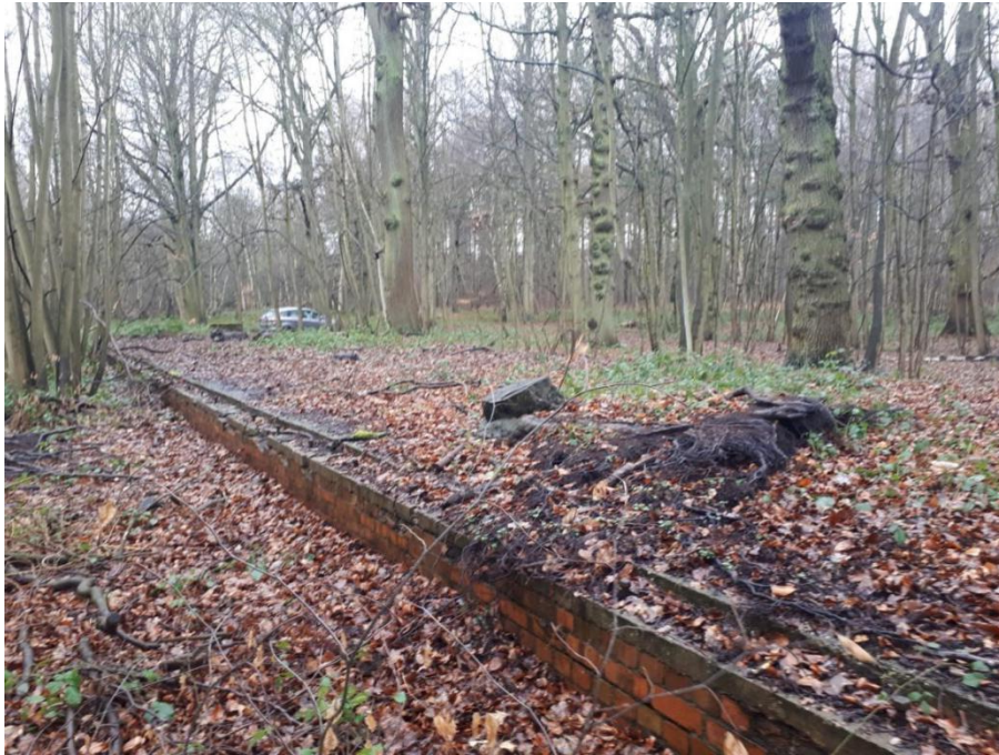
Photograph J_1: Remains of a brick and concrete military building railway platform. In Thoresby North Woods, former ammunitions store. Part of a railway system for transporting ammunition.
