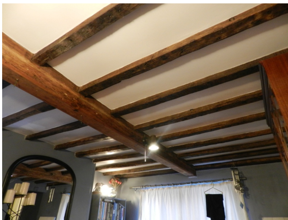
Fig 24 Timber joists and beam in the dining room of Arundel Cottage, looking south-east
