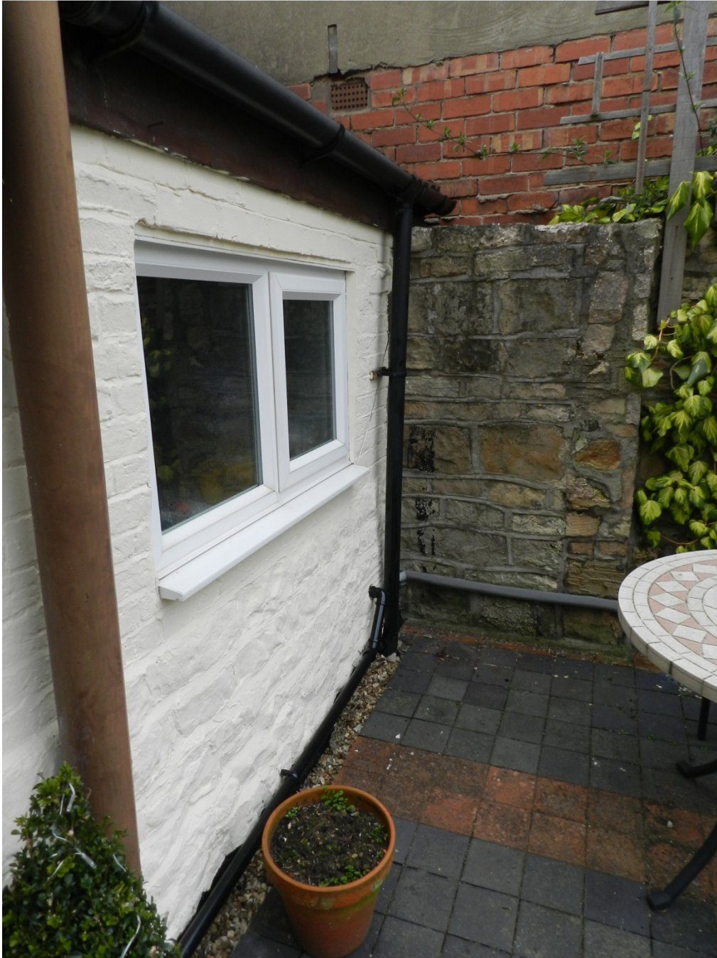
Fig 14 South elevation of the laundry of Brammer Farmhouse and the west elevation of Stone Wall 3, looking north-east
