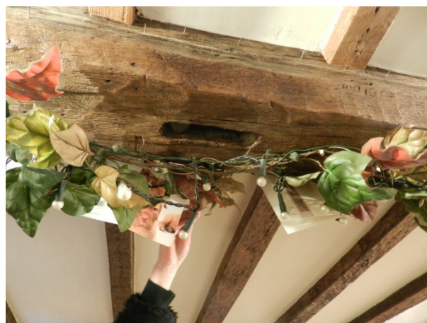
Fig 19 Empty mortice hole in the beam of the kitchen of Arundel Cottage, looking south-east
