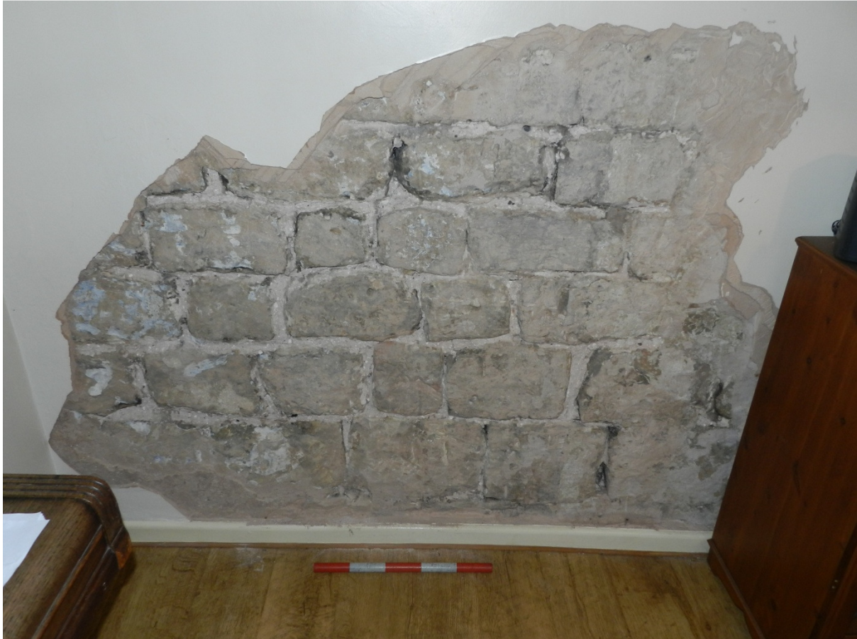
Fig 12 A section of removed plaster on the north wall of the living room of Arundel Cottage revealing the ashlar masonry of Stone Wall 2, looking north
