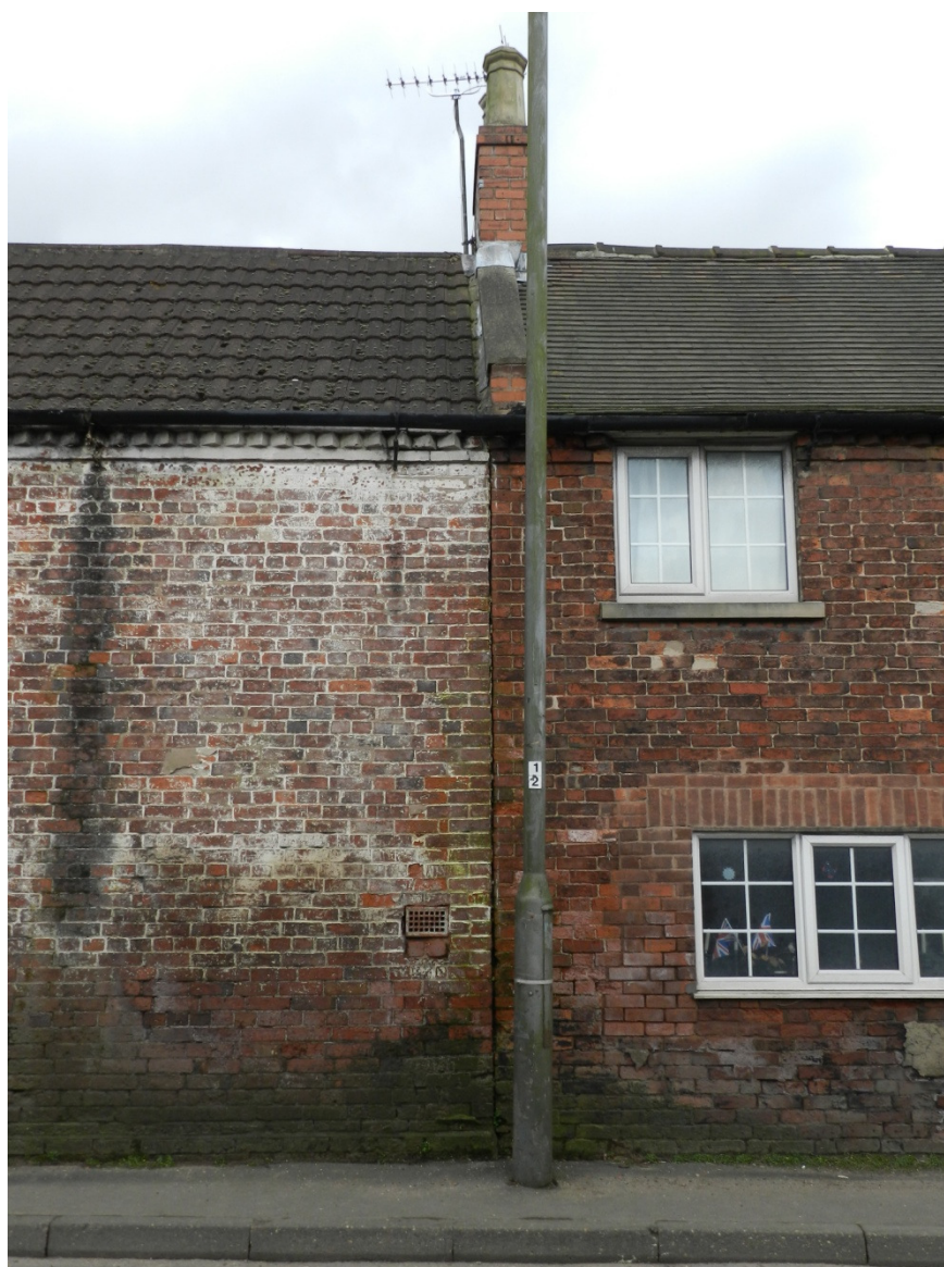
Fig 21 Straight joint between the Phase 2 single cottage (right) and the Phase 3 extension (left) of Arundel Cottage, looking south
