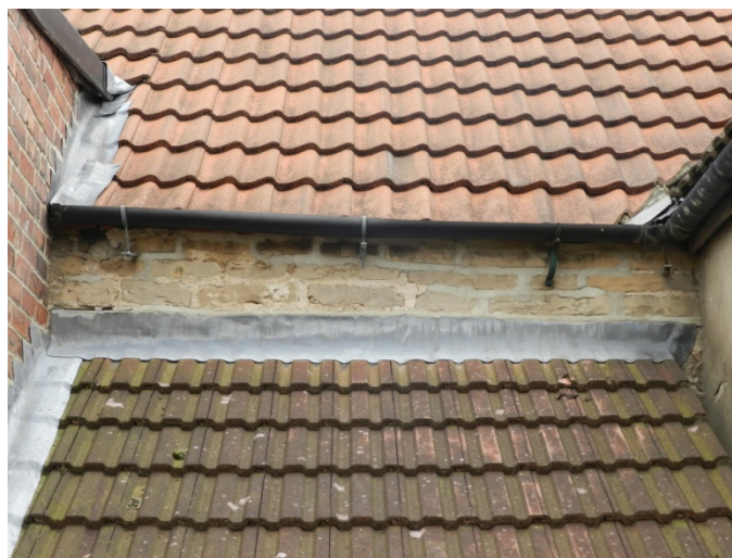
Fig 11 Stone Wall 2 above the roof of the laundry of Brammer Farmhouse, looking north
